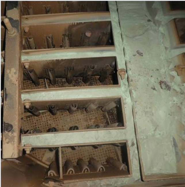
Before Chemical Clean
